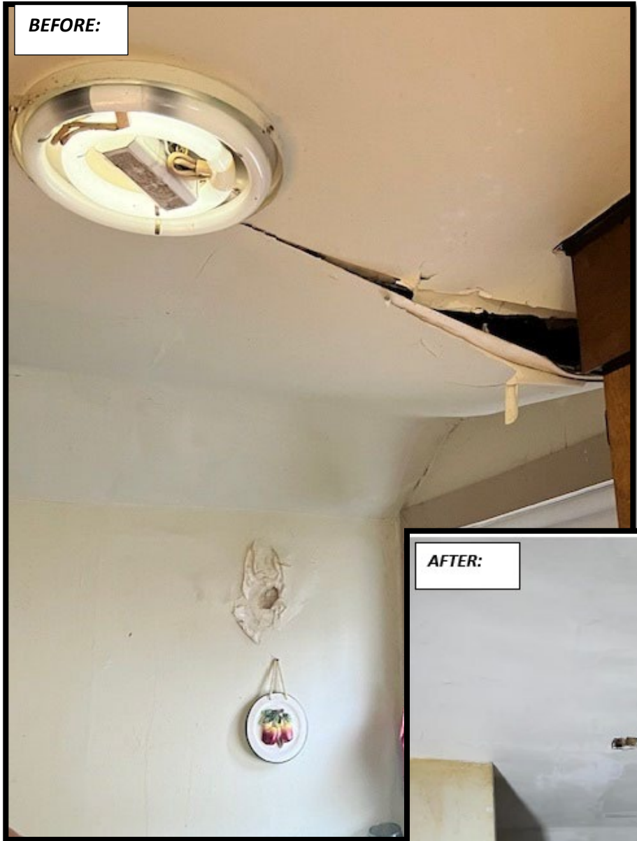
Kitchen ceiling under bathroom:
