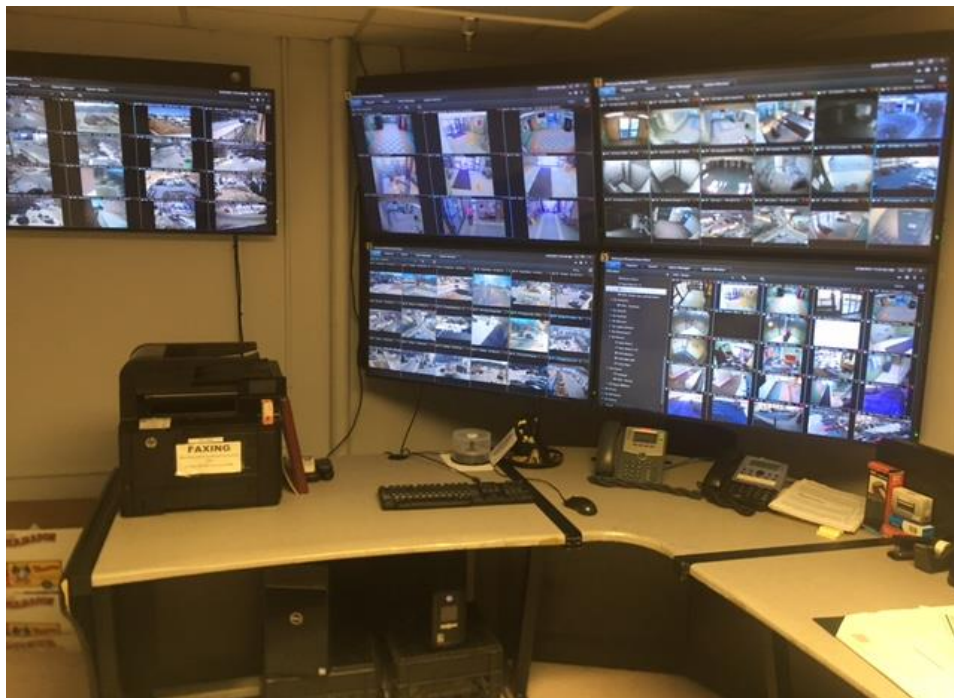
Central Security Dispatch Monitor Station
